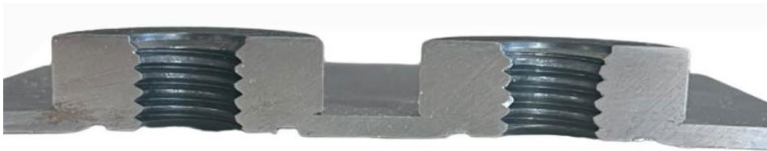
Figure 2. Cross-sectional view of the joint, showing the interlocking features between the clinch nut and the sheet metal after the clinching process
